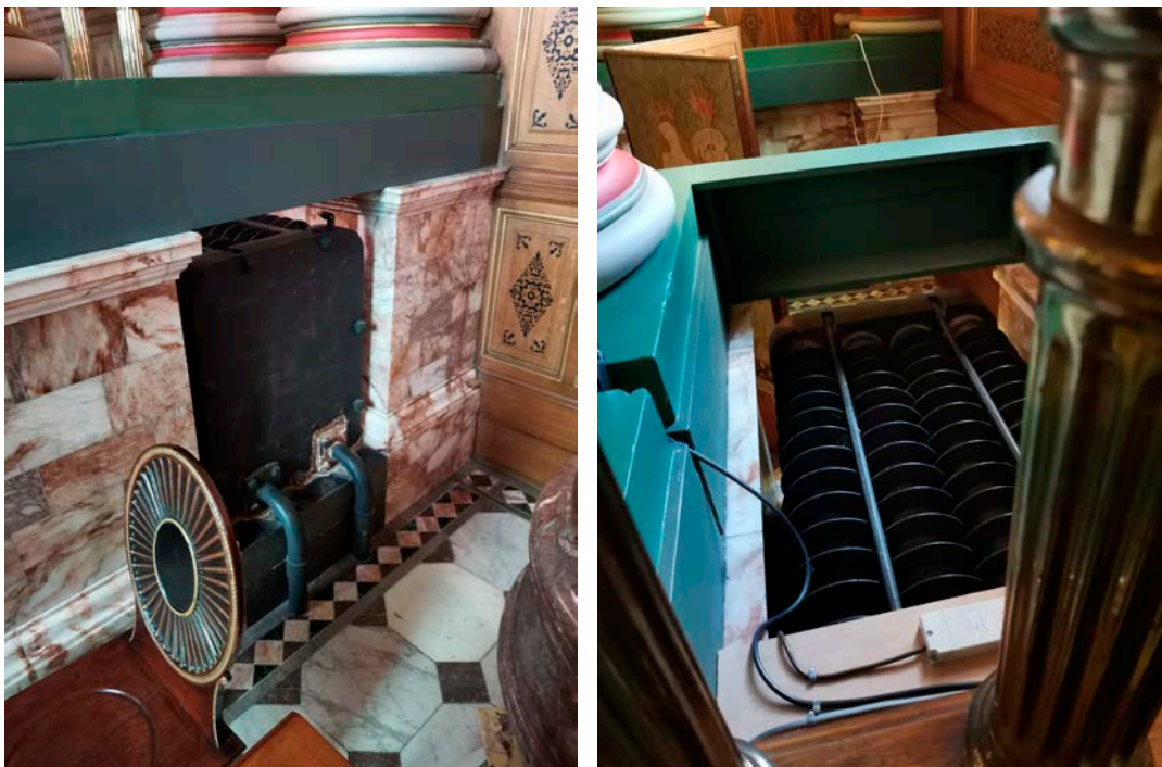
Figure 26: Historic radiators within the chapel.
