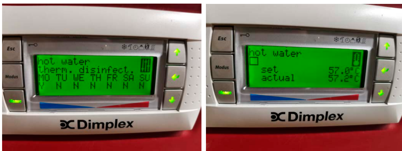
Figure 27: The WSHP control panel for the thermal disinfection cycle (left) and the hot water temperature (right).
