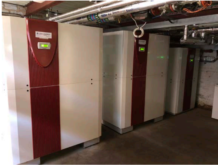
Figure 15: Dimplex WSHPs in the plant room.
