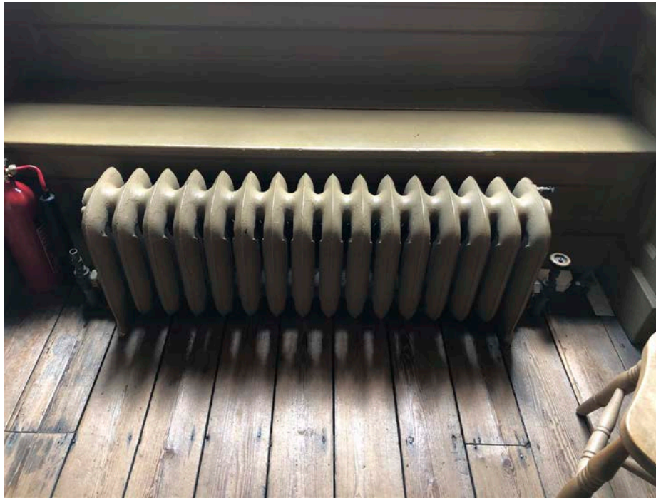
Figure 31: Cast iron radiator at Site 5.
