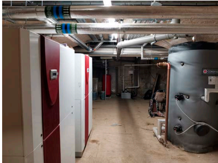
Figure 22: Dimplex SI 75TU WSHPs in the basement plant room at Site 4.
