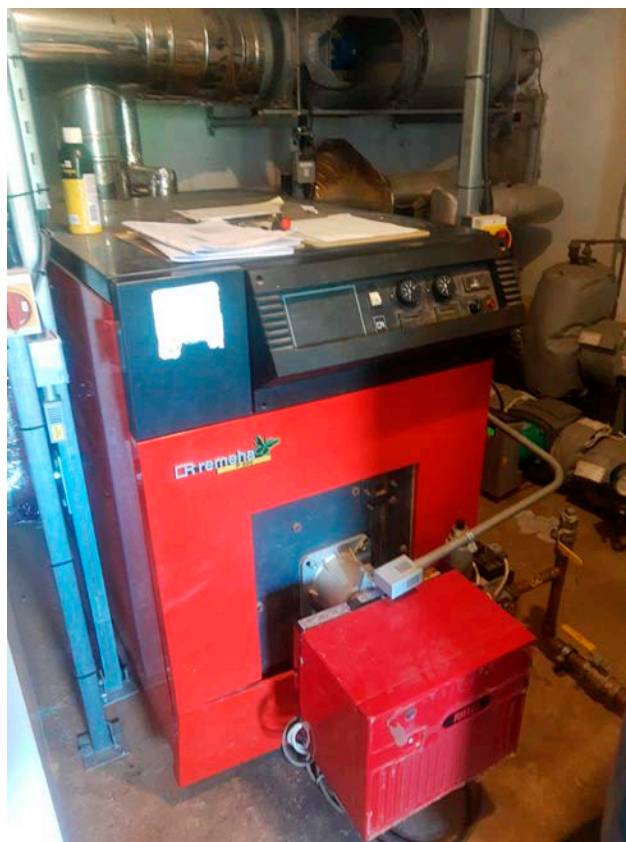
Figure 30: Existing oil boiler, which was repurposed to LPG.
