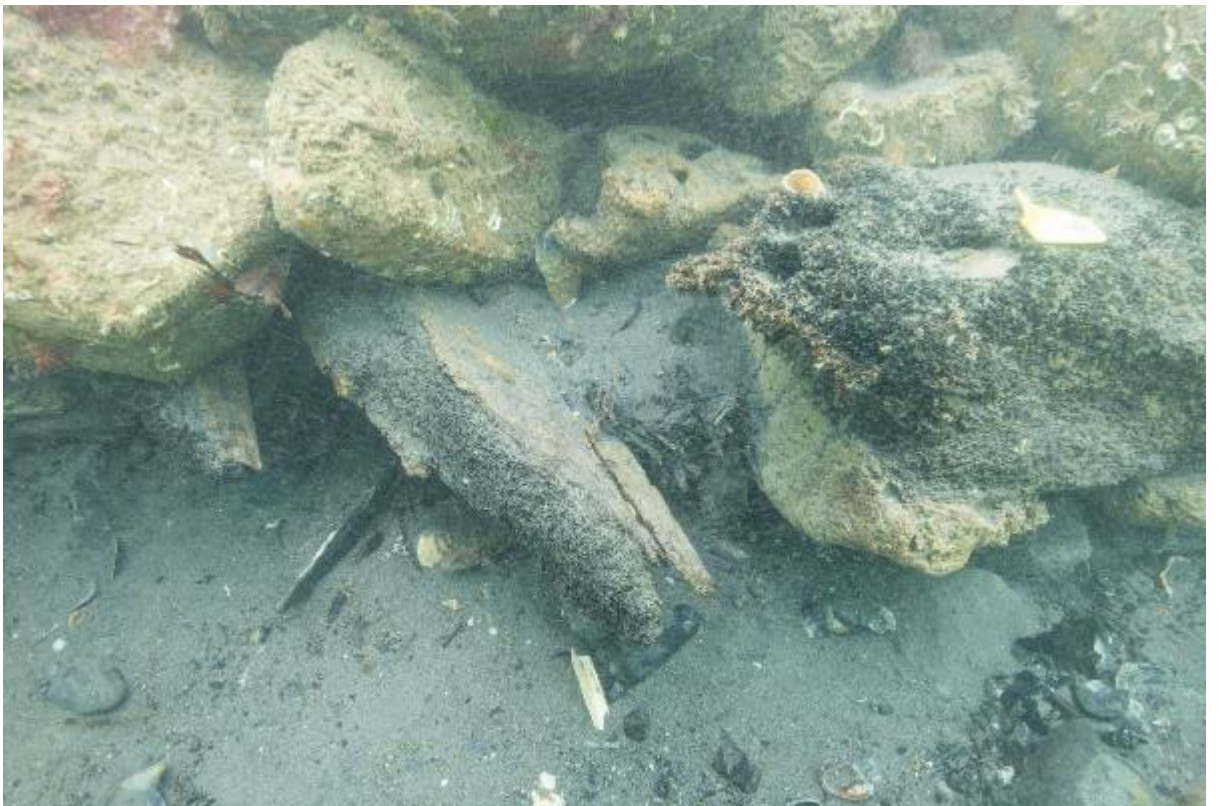
Figure 9. Frame and S10 showing significant wood borer damage.
