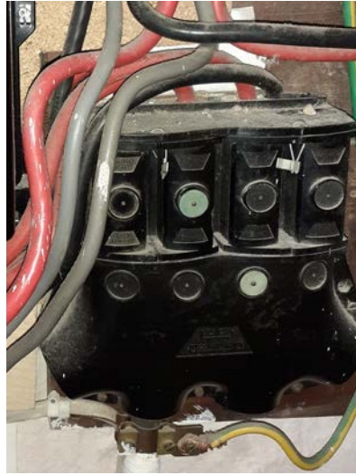
Figure 74: Electrical cut out and fuse housings.
