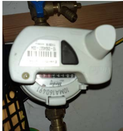
Figure 22: Church water meter (left).
