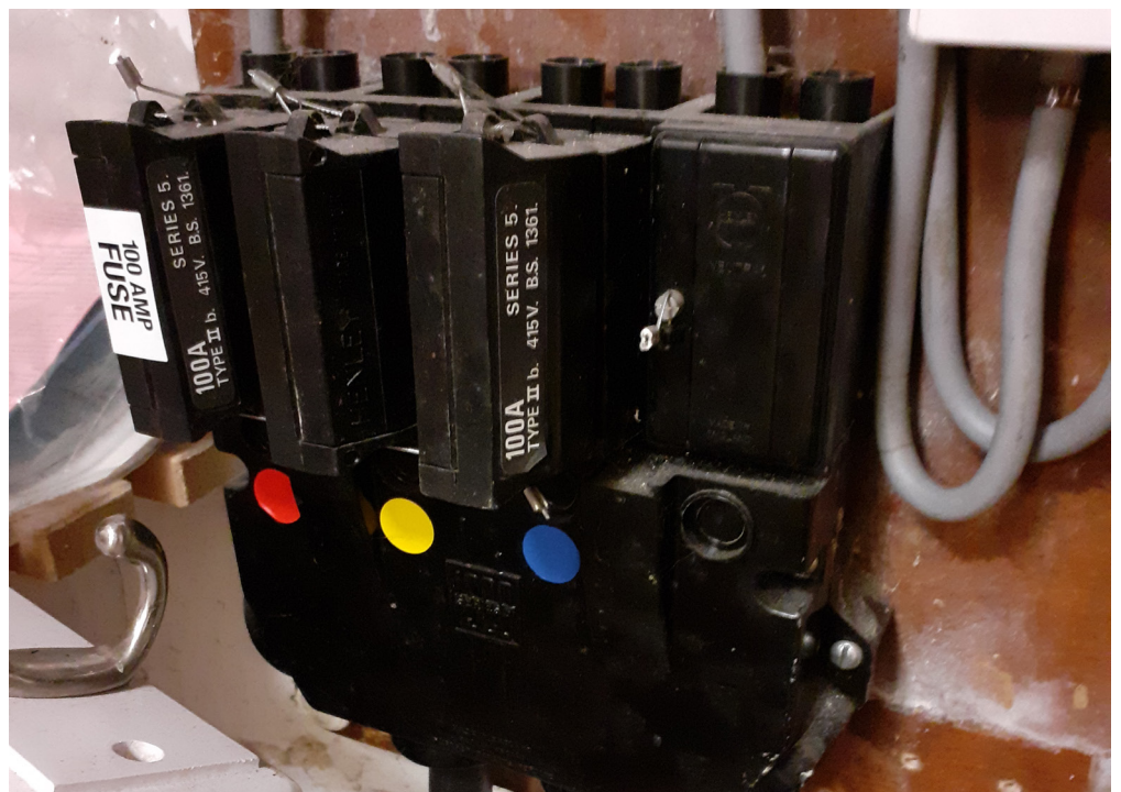
Figure 32: Electrical cut out and fuse housings.
