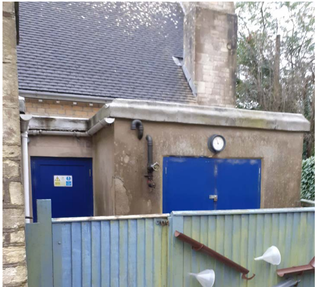
Figure 30: Plant room and oil tank room.
