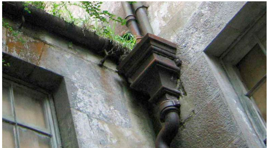
Figure 15: Rainwater overflowing from a partially blocked gutter and hopper head was indicated by the algae staining the wall. In addition, the back of the hopper had corroded and water was leaking into the wall through open joints.
