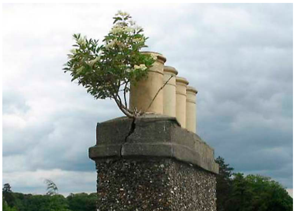
Figure 20: The roots of a shrub growing in a chimney stack cause structural damage and allows water penetration. These problems will get worse as the plant grows.
