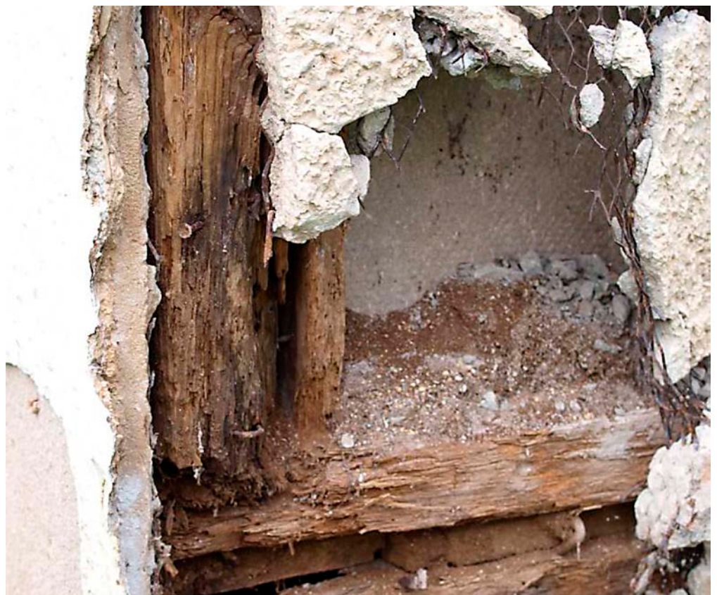
Figure 21: This timber frame was covered by an impermeable cementitious render on metal mesh. Fine shrinkage cracks allowed moisture to penetrate. In addition, condensation occurred on the cold interior surface of the render. Trapped moisture at the interface between the frame and the render caused the timber to decay.
