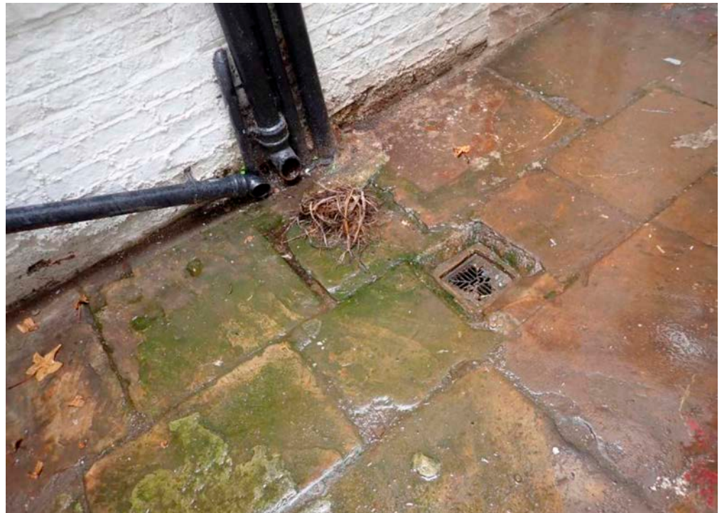
Figure 19: The ground floor in this building is at the same level as the external ground level, so it is essential that the external area is well drained. Unfortunately, water discharging from the rainwater pipe does not reach the gully because of the unevenness of the paving. Instead, it soaks into the joints between the slabs, allowing vegetation to grow and saturating the ground beneath. Moisture then rises within the wall.
