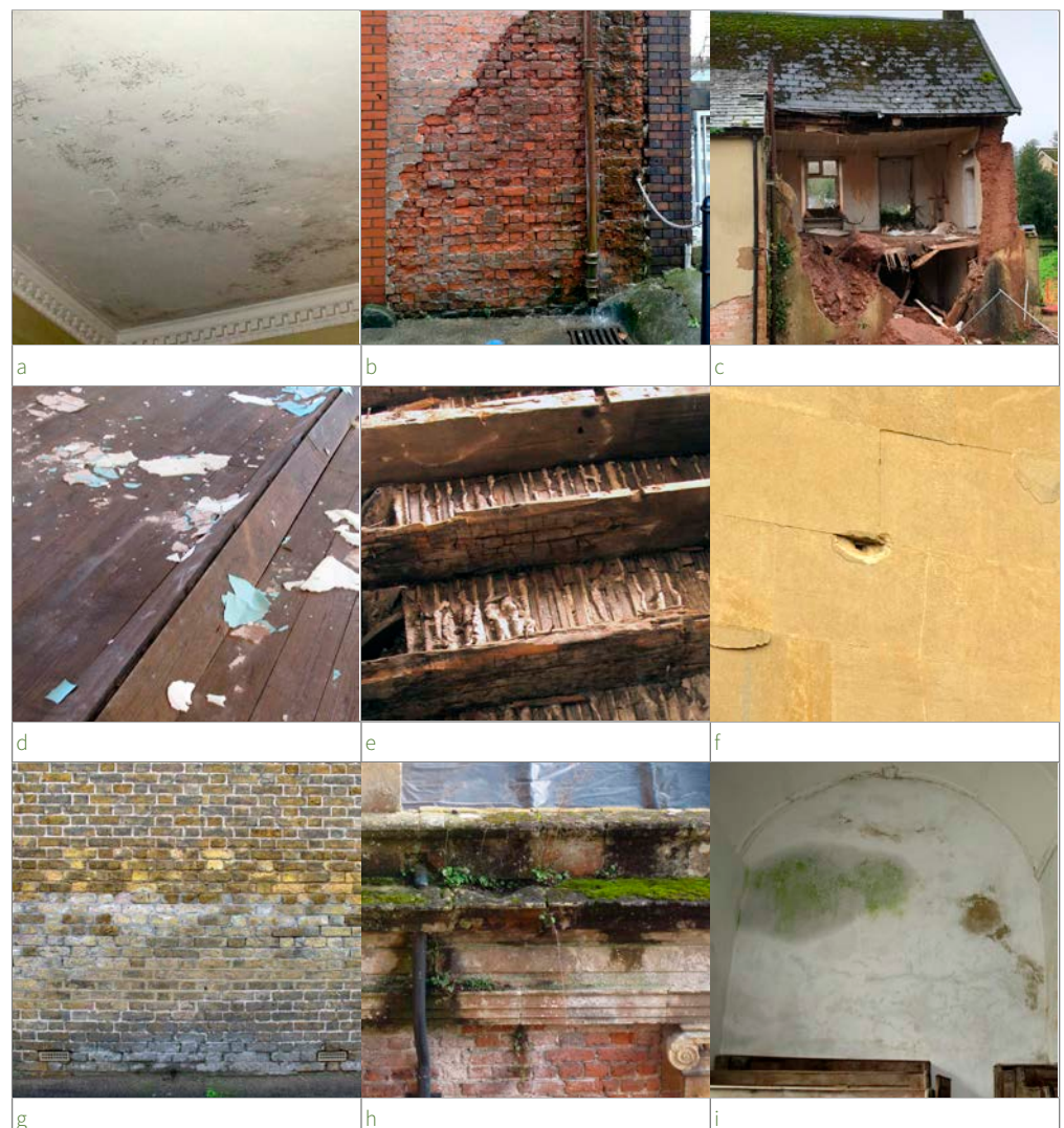
Figure 3: Deterioration and damage caused by excess moisture: a. Mould growth on internal surfaces. b. Freeze/thaw damage to brickwork saturated by blocked rainwater pipe. c. Collapse of earthen walling caused by water trapped by impermeable surface finishes. d. Warping and buckling of floor boards saturated by flooding. e. Timber decay and infestation. f. Spalling of masonry caused by corrosion of embedded iron cramps. g. Salt crystallisation damage to brickwork. h. Colonisation of surface by algae, moss and plants. i. Damp patches – internal finishes disfigured and damaged.
