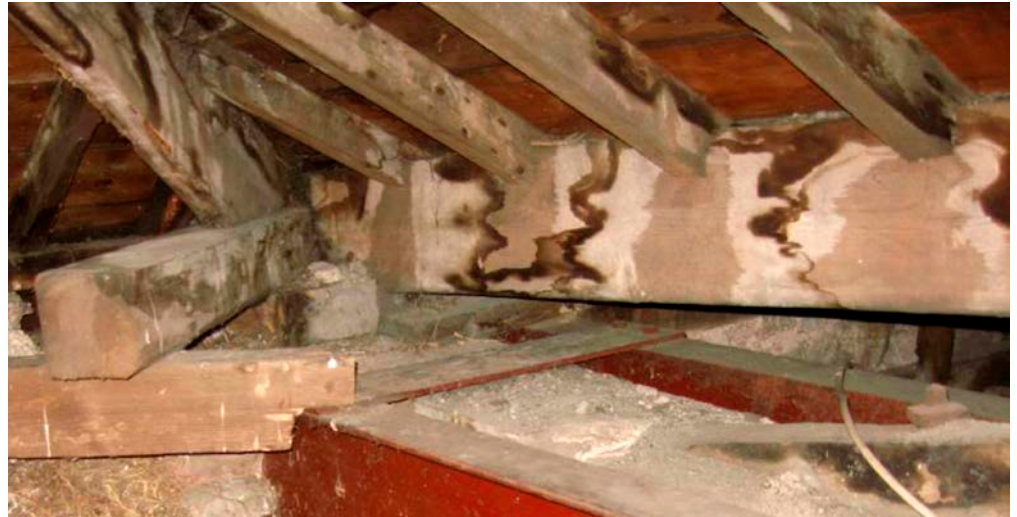
Figure 35: Damp staining on roof timbers might suggest the need for assessment with a moisture meter, but superficial chemical changes in the timber or contamination in the stained areas may result in erroneous readings.
