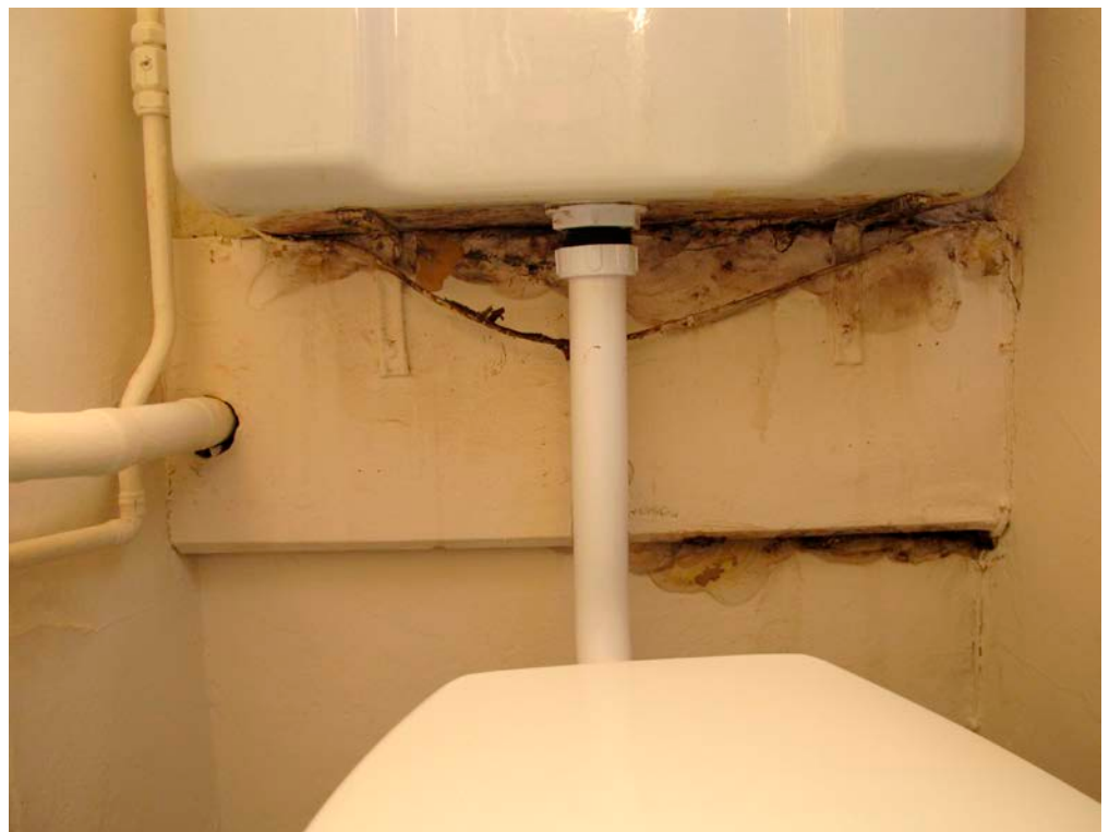
Figure 14: Water from a leaking cistern has resulted in fungal decay in a timber pattress.
