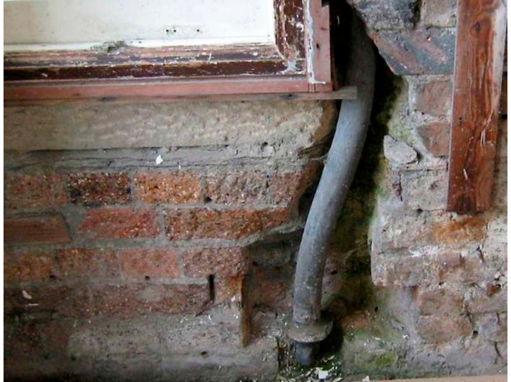
Figure 17: An old lead internal rainwater pipe revealed when wall linings were removed.
