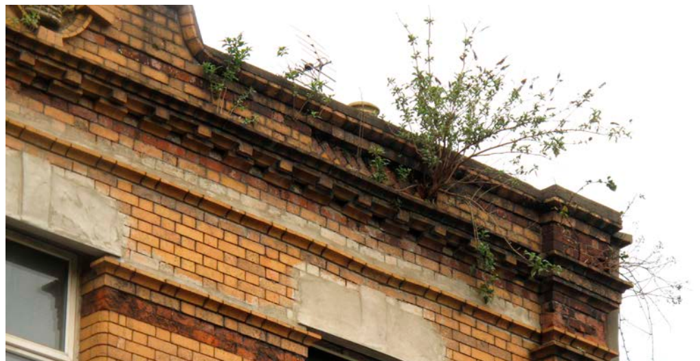
Figure 16: Height and restricted access can make gutter inspection and clearing difficult and expensive. However, if vegetation is visible from ground level, it is likely that rainwater will be finding its own way down through the building.
