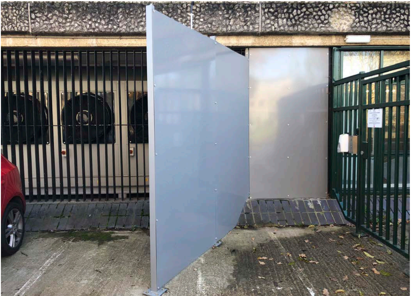
Figure 22: Barrier to divert flow of cold air from the evaporators away from the nursery entrance.
