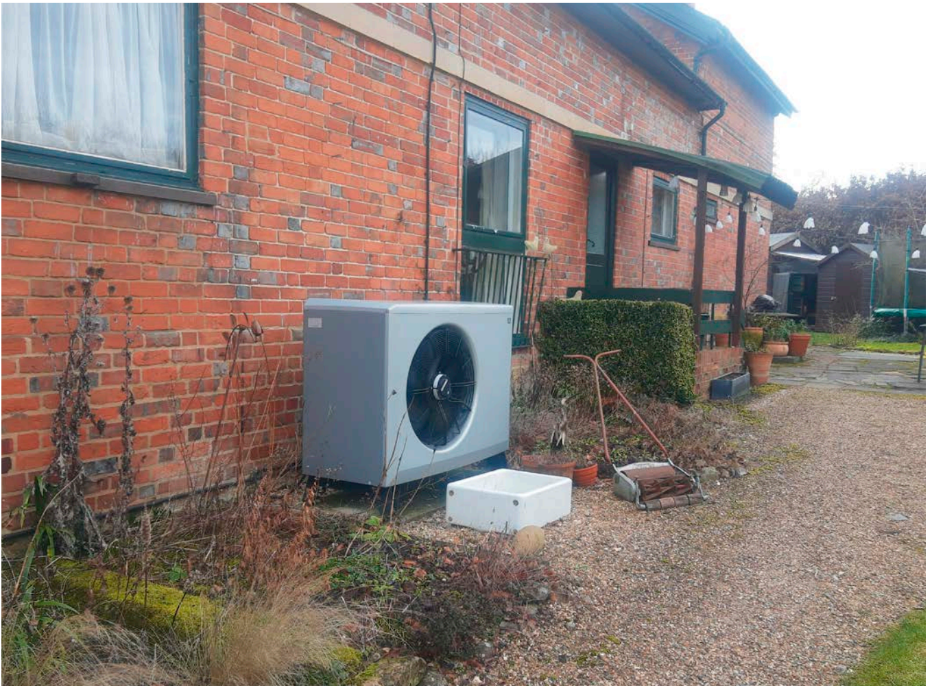
Figure 24: ASHP at Site 4b.
