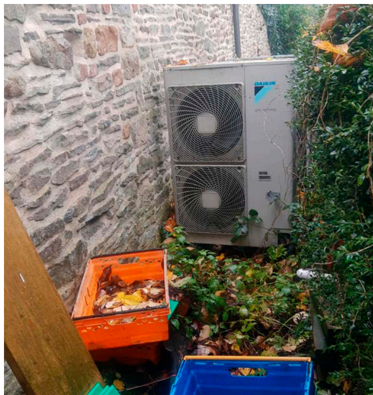
Figure 10: ASHP at the rear of Site 1 workshops.
