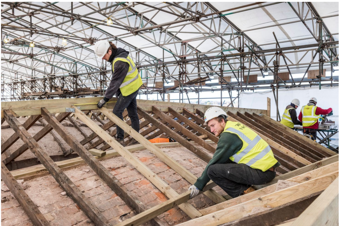
Figure 2: Prince's Foundation trainees learn new skills on the roof of the Main Mill [© Historic England Archive, Steven Baker]
