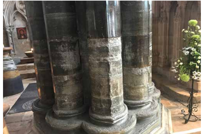
Low level decay on a Purbeck Marble column at Lincoln Cathedral.
