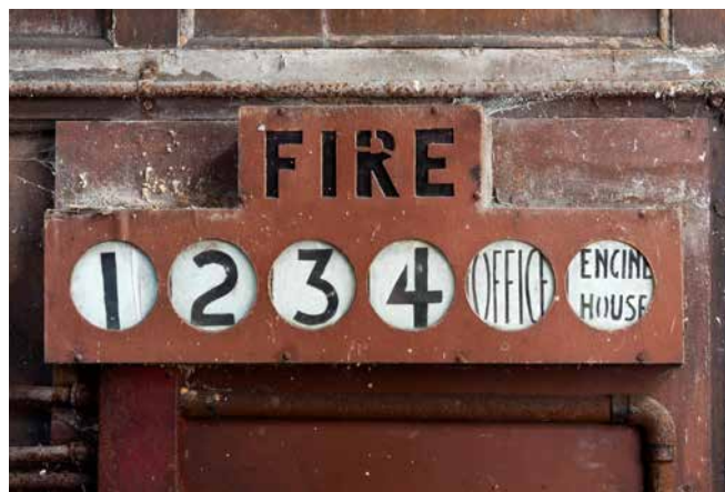
The old fire alarm panel at the Waterloo Mills, Bradford.
