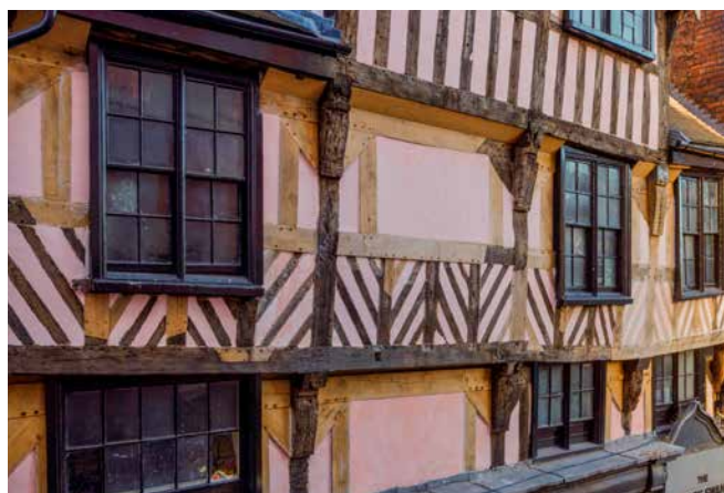
An early 17th-century jettied timber-framed building in Wakefield after repair works in 2023.
