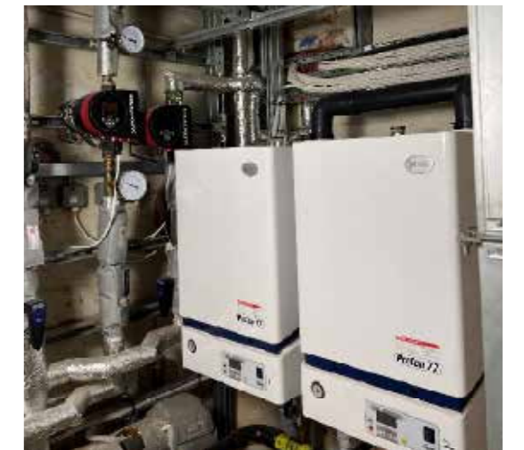
Figure 3-3: Basement plant room housing 2no condensing gas boilers
