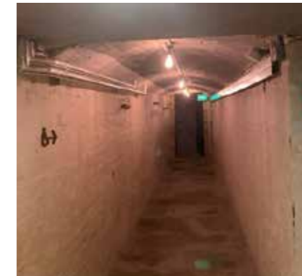
Fluorescent fittings within basement corridor
