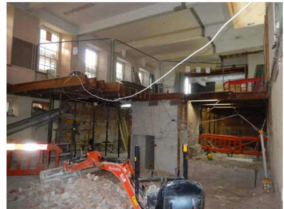
Cafe and shop during the 2018 refurbishment works Image source: Philip Hughes Associates
