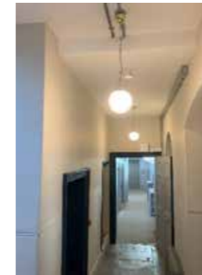
Pendant fittings in circulation areas
