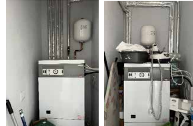
Electric boilers to flats
