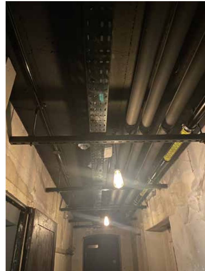
Services routes through the basement
