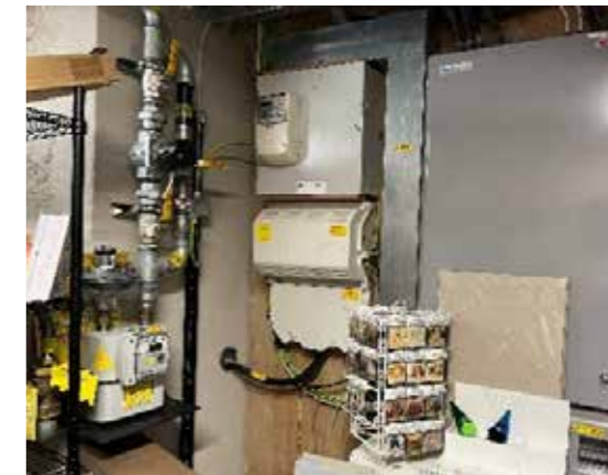
Incoming supply and adjacent switch panel
