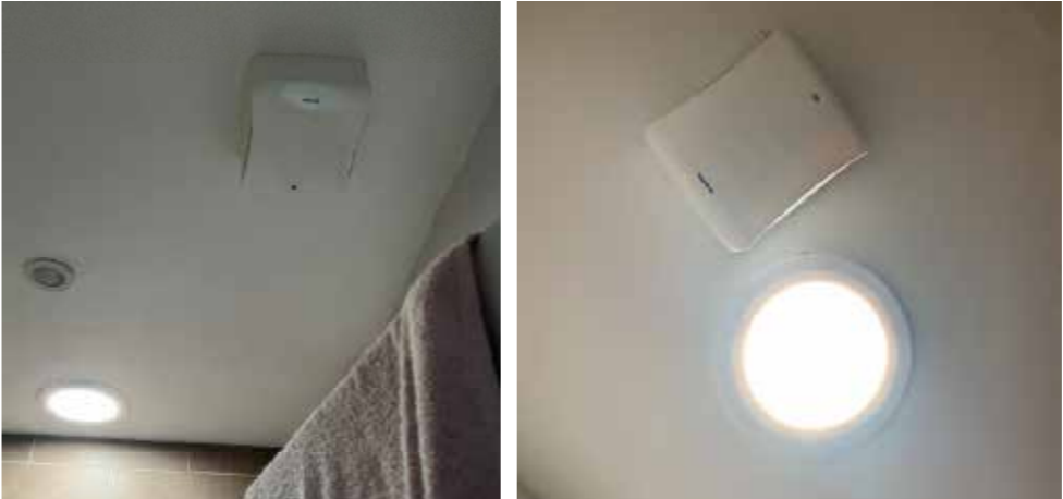
Ceiling mounted Vent-Axia extract fans in flat bathrooms
