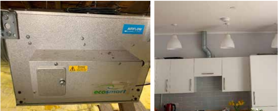
Right: Un-labelled extract fan in roof void. Left: Ventilation ductwork from kitchen cooker hood
