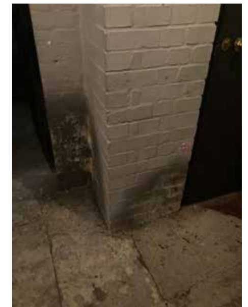
Damp in basement
