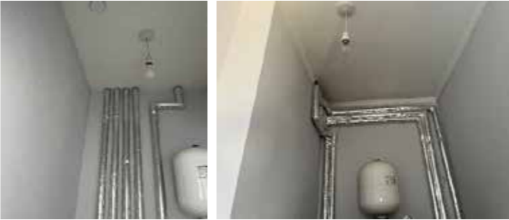
Insulated pipework to flats
