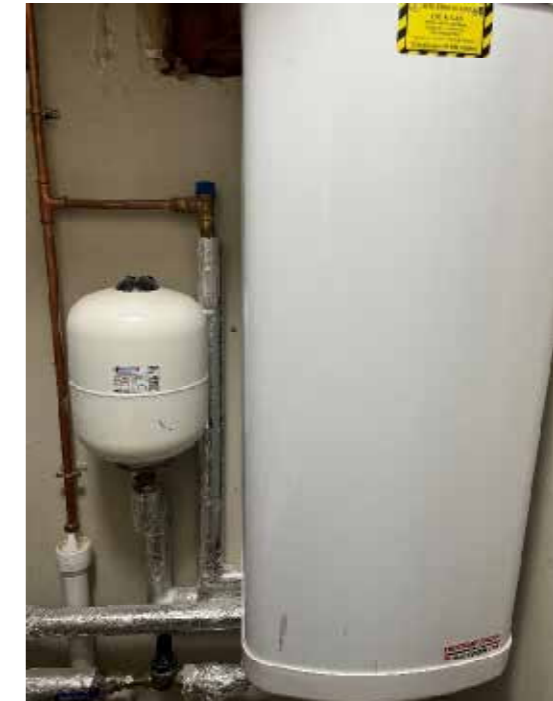
Cafe store cupboard housing an electric water heater
