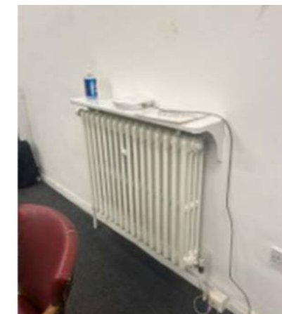
Column radiator in multi-purpose area
