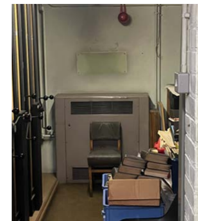
Fan assisted heater in basement archives
