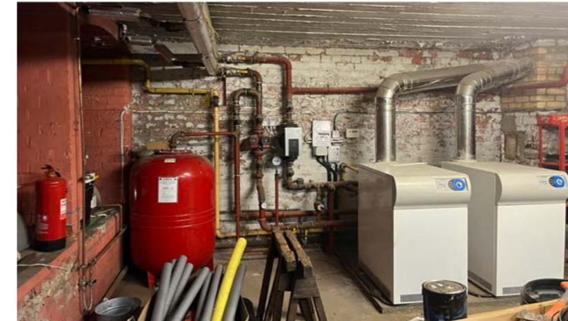
2x gas boilers, expansion set, twin head pumps in basement
