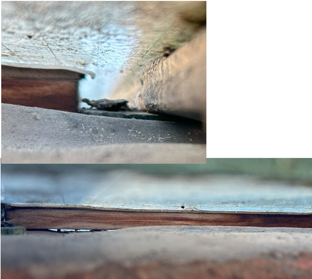
Some leakage from all three "Greenhouses" between the lower edge of roof glass and frame (which were the only locations easily checkable). Seals shrunk or a gap was intentional.
