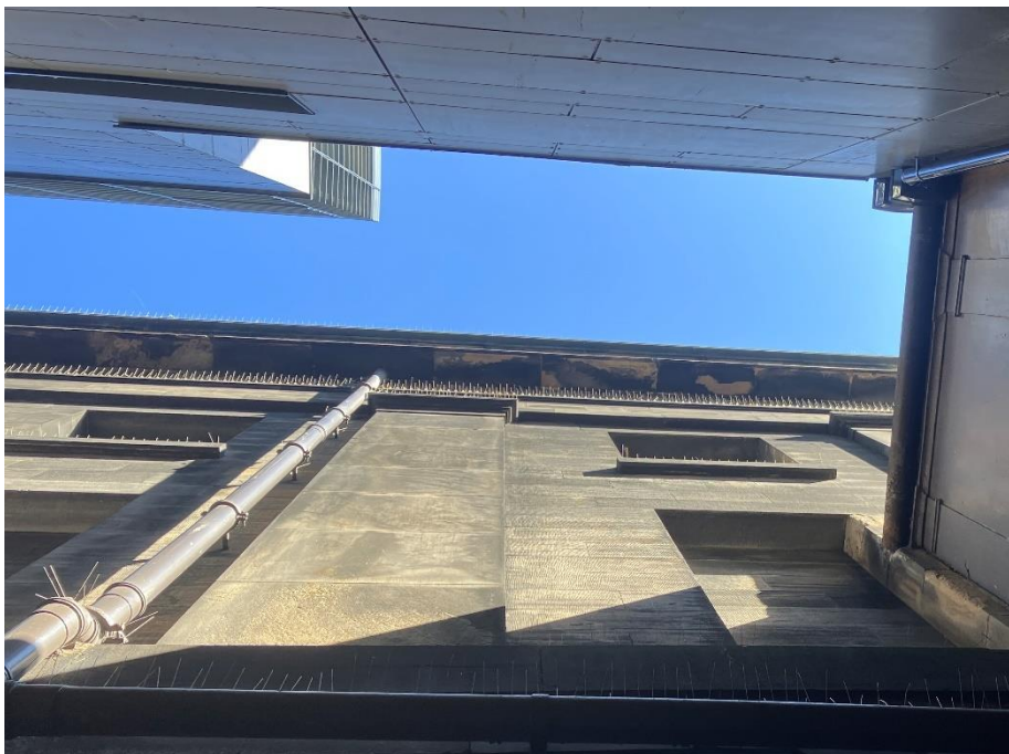
Photograph 11: West flank elevation – water staining to cornice.
