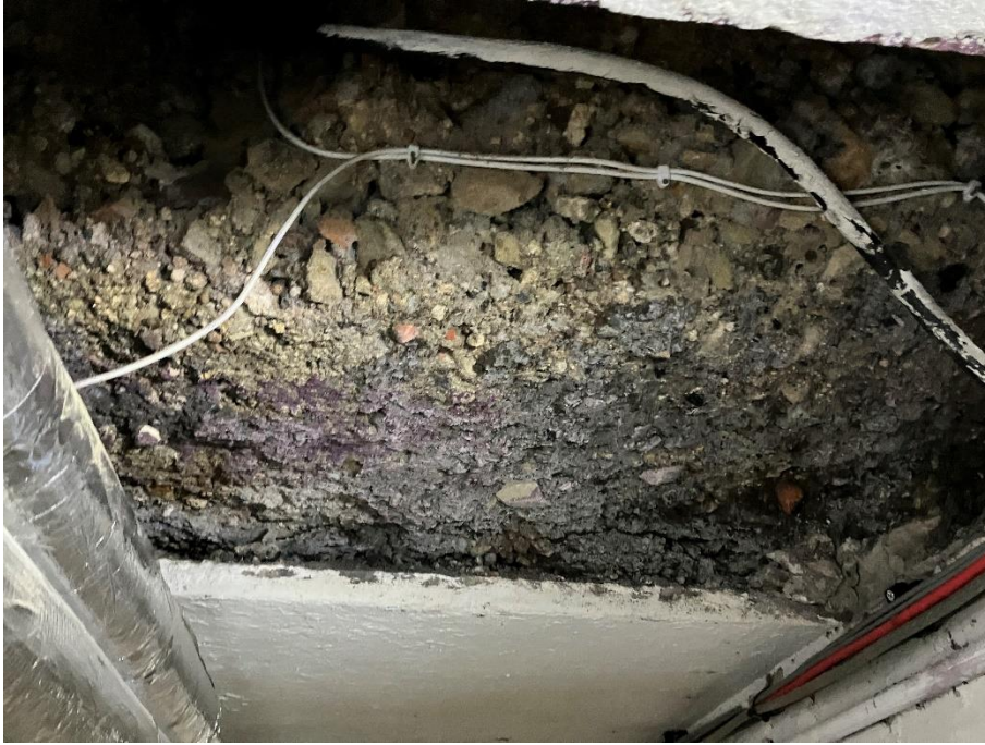
Photograph 18: Basement – failed roof to boiler room access tunnel
