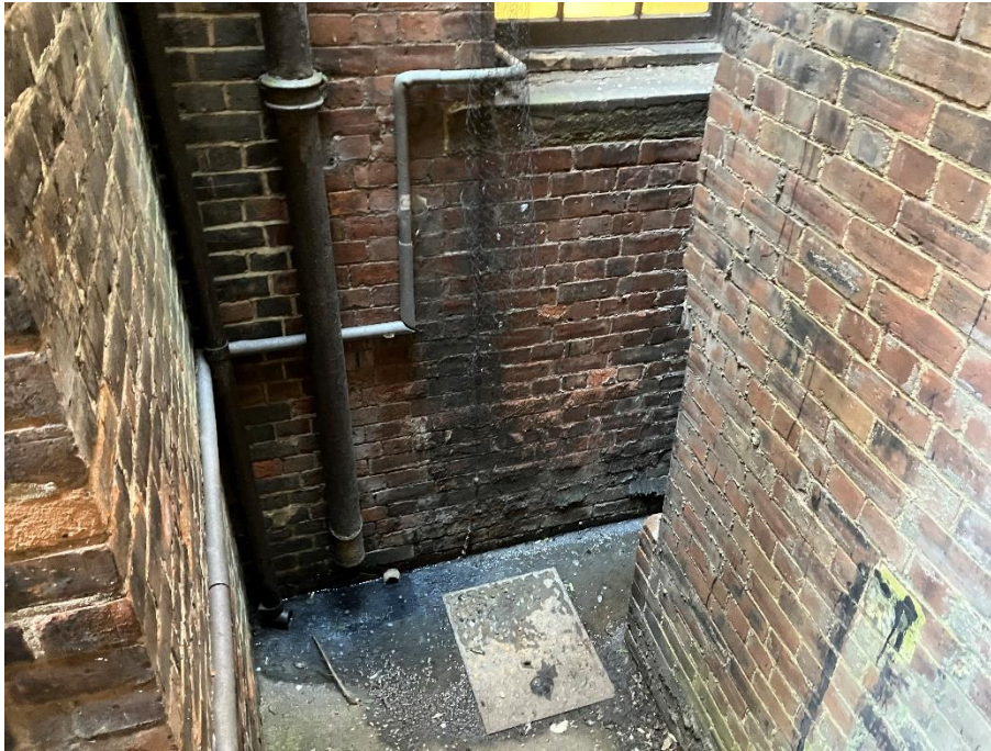
Photograph 13: Rear (south) elevation – RWP discharging onto ground externally
