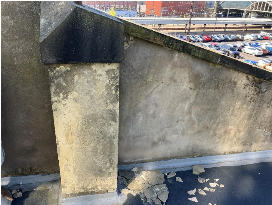
Photograph 8: Typical example of failed render at roof level.
