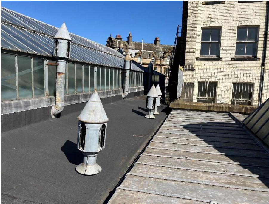
Photograph 6: Junction and shallow drainage channel between lead and felt finishes.
