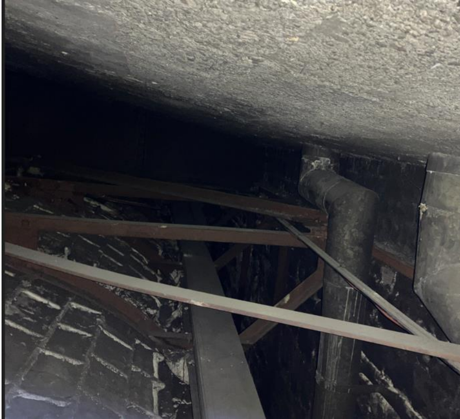
Photograph 2: View within Main Library roof void showing steel framing supporting fibrous plaster coved ceiling and concrete slab roof deck over.
