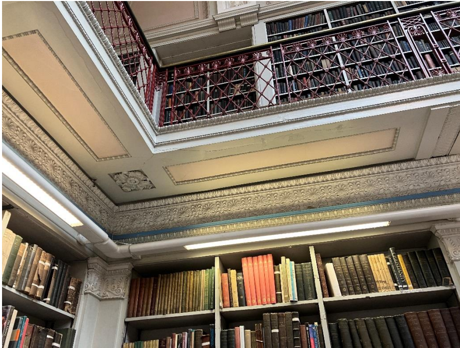
Photograph 23: Typical example of plaster cracking to the fascia and soffit of the library galleries
