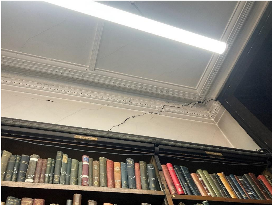
Photograph 21: Ground Floor – Reading & Silence Room, crack at north-west corner
