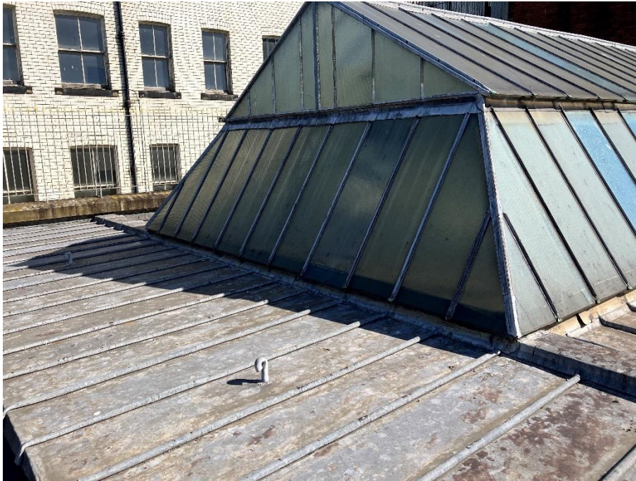
Photograph 3: Reading Room 'glasshouse and leaded flat roof deck. A structural beam supporting the roof lights and glass house can be seen spanning N-S between the external walls and covered by the leaded upstand.
