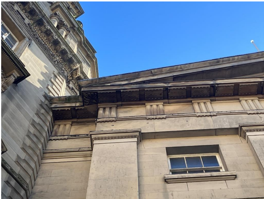
Photograph 9: Front elevation - water staining at upper north-east corner.
