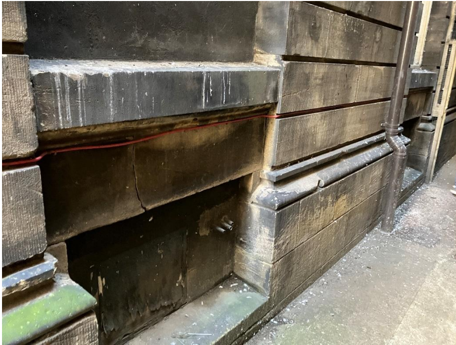
Photograph 10: West flank elevation – cracked lintel.
