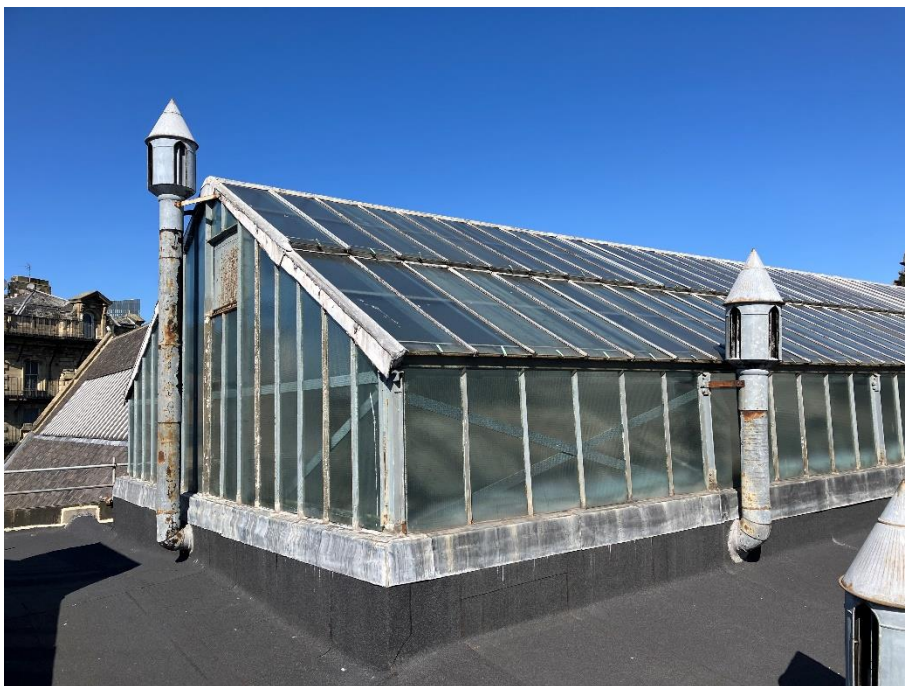
Photograph 1: View of current steel glasshouse frame over roof light openings and felt roof coverings. No primary steel structure is visible.
