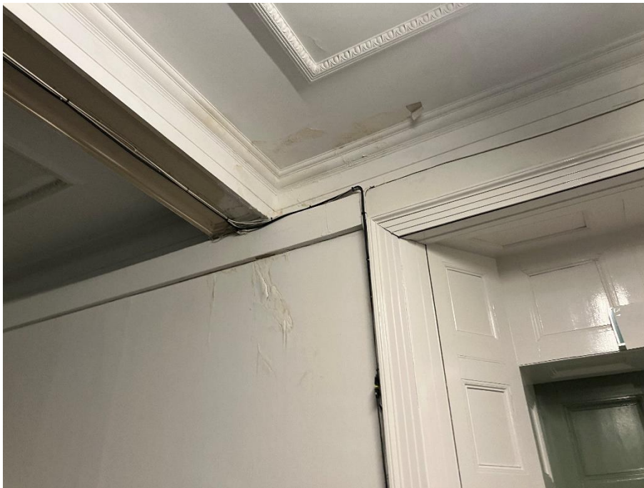
Photograph 19: Ground Floor – Loftus Room, water damage around probable beam bearing
