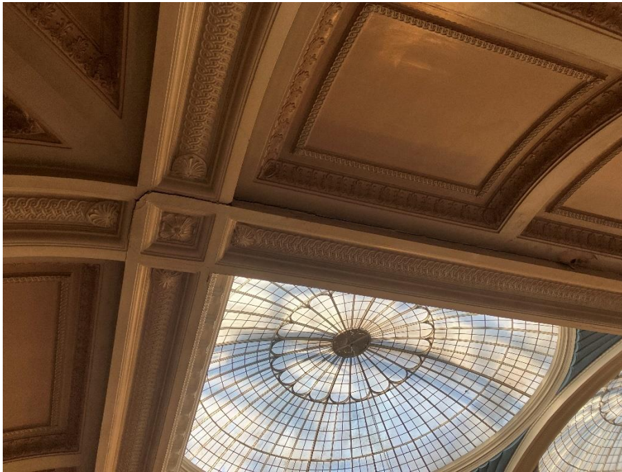
Photograph 24: Main library – example of failed and detached ceiling plaster
