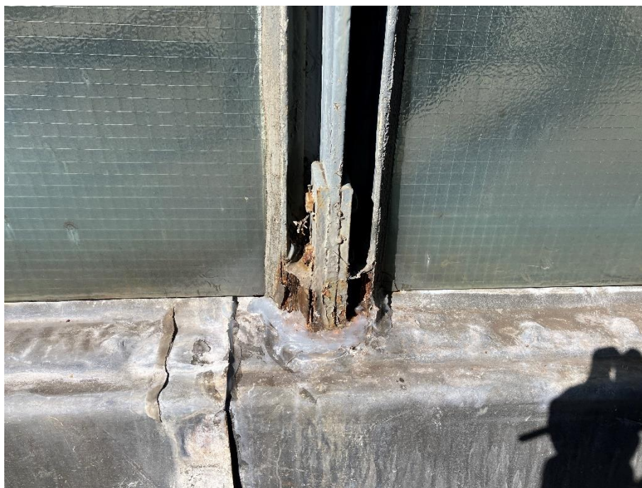
Photograph 6: Typical example of corrosion to base of steel framing
