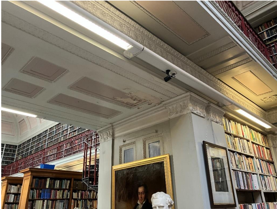
Photograph 25: Water ingress between the Main Library and Reading Room
