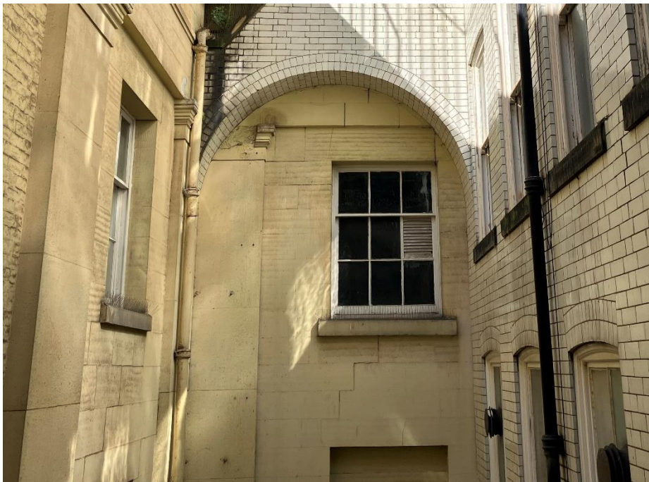
Photograph 16: Stepped cracking to masonry in the courtyard.
