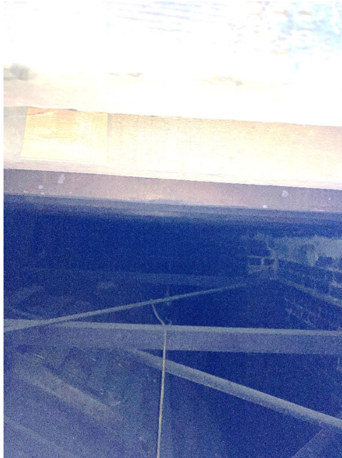
Photograph 4: View within Reading Room roof void showing covered ceiling plaster, secondary steel structure and timber joist deck over.
