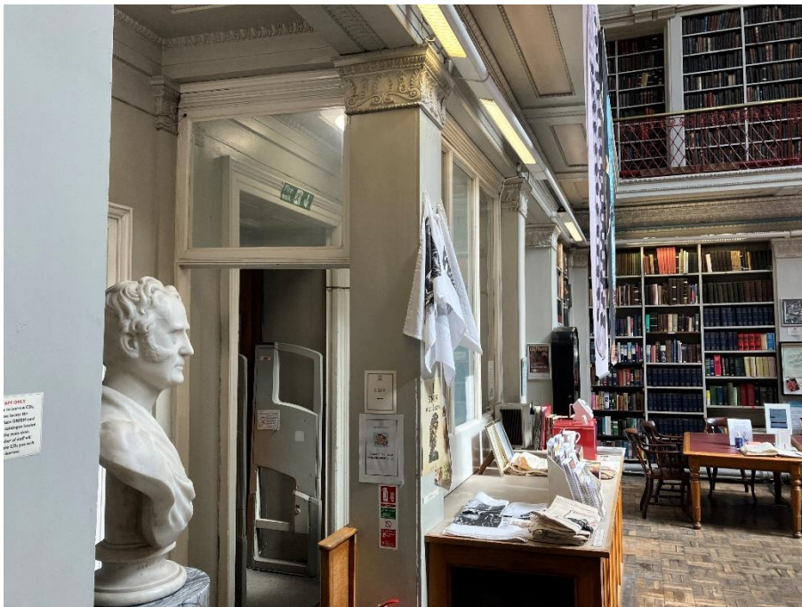
Photograph 22: Main Library – apparent settlement of columns supporting the gallery
