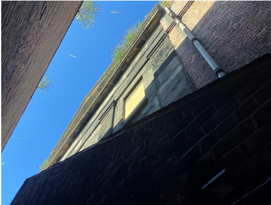
Photograph 12: Rear (south) elevation - plant growth and water staining to pediment.
