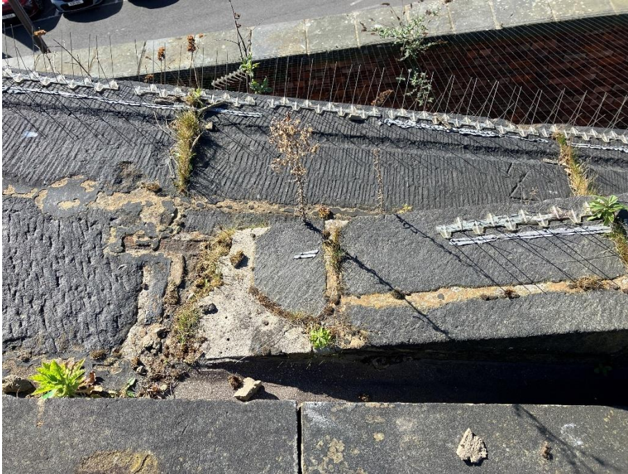
Photograph 7: Typical example of roof level masonry showing open joints, vegetation growth and an exposed iron cramp.
