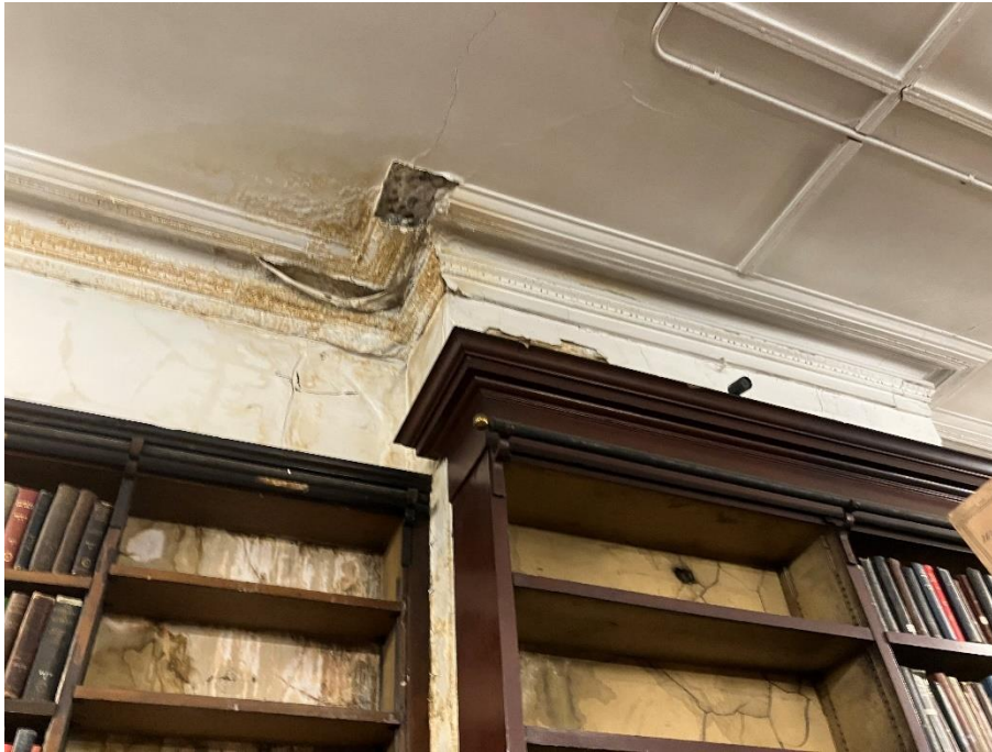
Photograph 20: Ground Floor – Reading & Silence Room, water damage at eastern end
