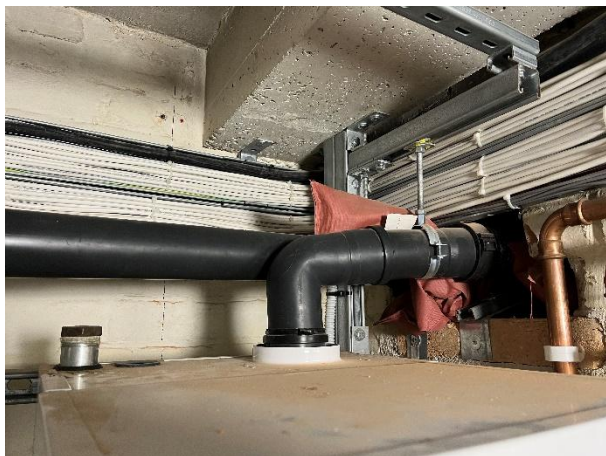
Figure 5-6 Boiler flues entering existing chimney
