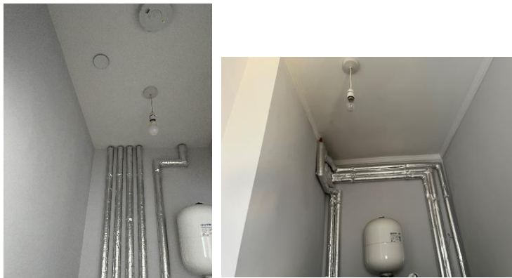
Figure 6-3 Insulated pipework to flats
