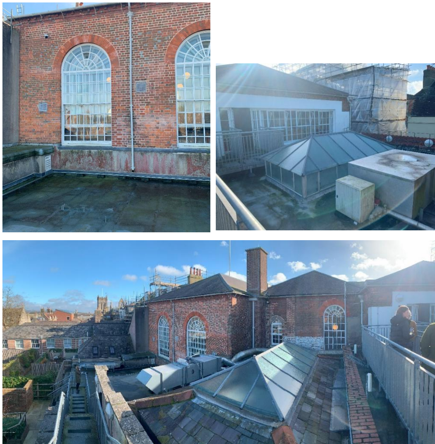
Figure 7-2 Images of flat roofs to the rear of the building showing the roof lanterns
