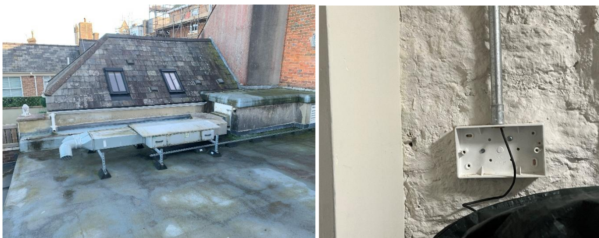
Figure 5-10 Left: MVHR unit located on low rear roof assumed to server basement museum areas. Access up to unit not possible. Right: assumed system controller location in store at basement level.
