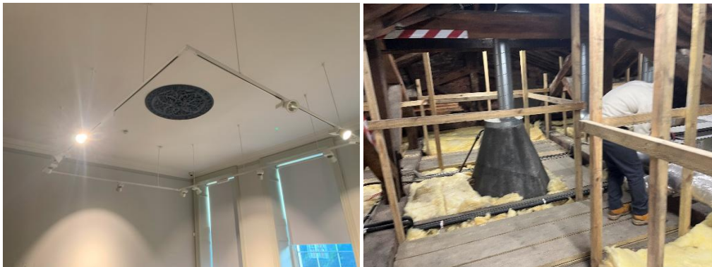
Figure 5-17 Left: Ornate ceiling grille in Grand Jury Room. Right: ductwork connection onto ceiling grille in roof void.
