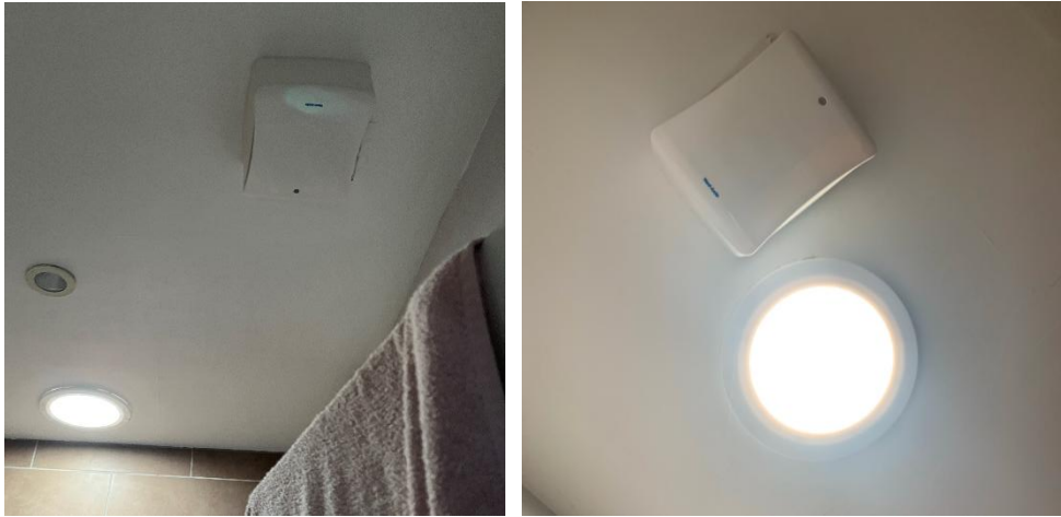
Figure 6-5 Ceiling mounted Vent-Axia extract fans in flat bathrooms
