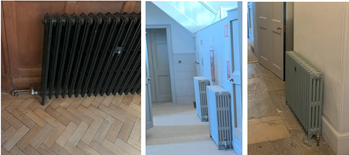
Figure 5-9 Cast iron radiators to Learning space (left), Crown court (middle) & circulation space (right)
