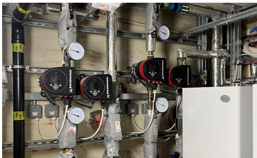
Figure 5-7 Heating pumps serving zones 1 & 2
