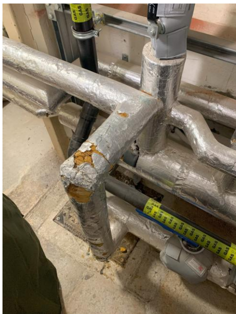
Figure 5-8 - Damage to pipework insulation in plant room
