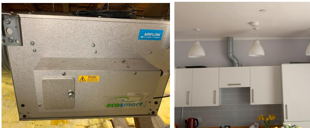
Figure 6-4 Right: Un-labelled extract fan in roof void. Left: Ventilation ductwork from kitchen cooker hood
