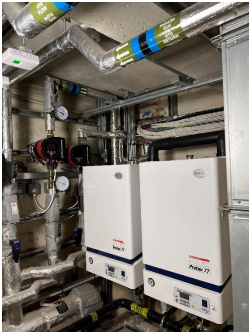
Figure 5-4 Boilers mounted on rear wall of plant room
