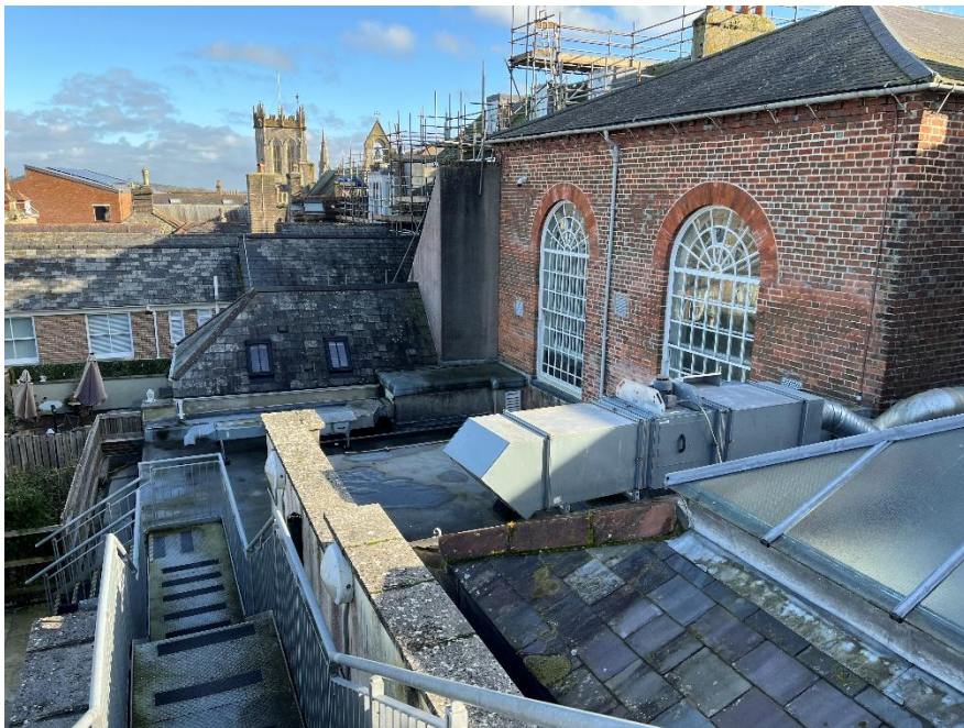
Figure 5-12 Cafe extract fan on low rear roof
