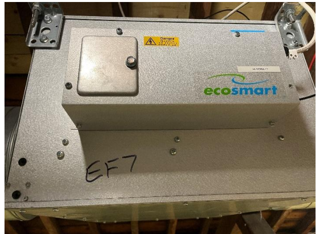
Figure 5-15 Extract fan EF7 located in roof void
