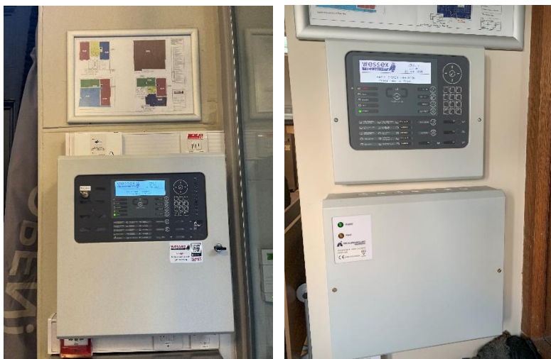
Figure 5-19 Left: Main fire alarm panel adjacent to main entrance. Right repeater panel located by the entrance from the car park to the rear of the building.
