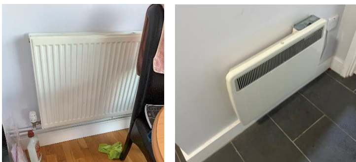
Figure 6-2 Left: LTHW panel radiator to flat. Right: Electric radiator to communal hallway
