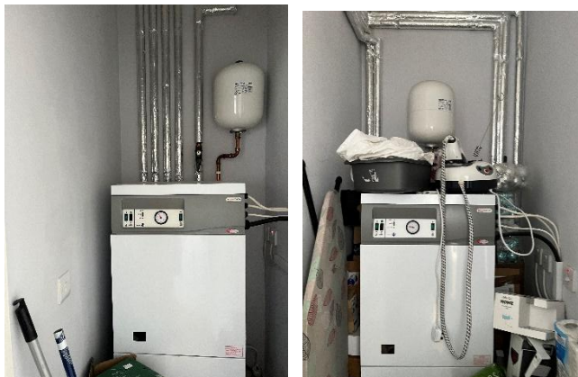
Figure 6-1 Electric boilers to flats
