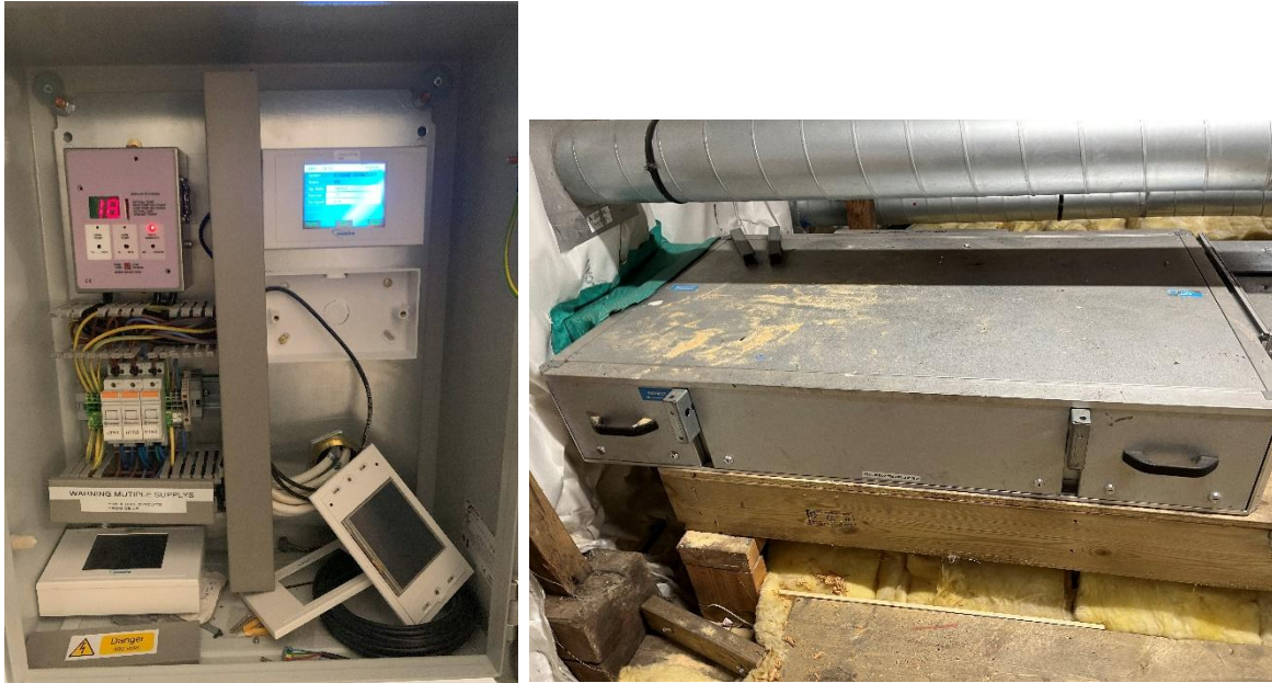
Figure 5-16 Right: Grand Jury Room fan controller disassembled (right bottom). Left: MVHR unit in roof void assumed to serve grand Jury room
