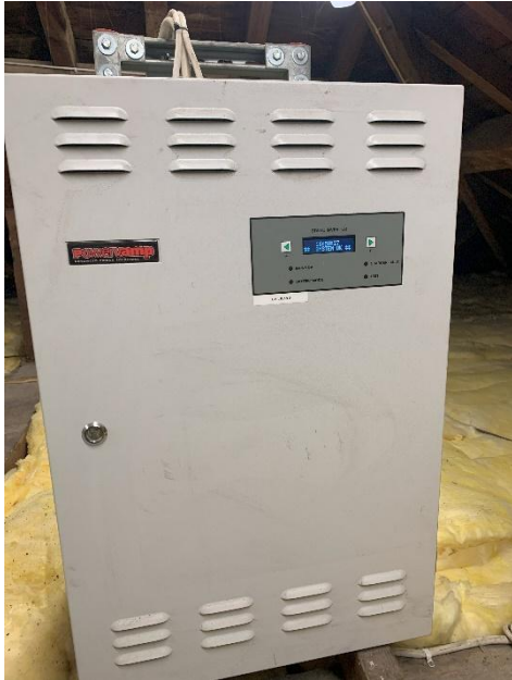
Figure 5-18 Static inverter located in roof void
