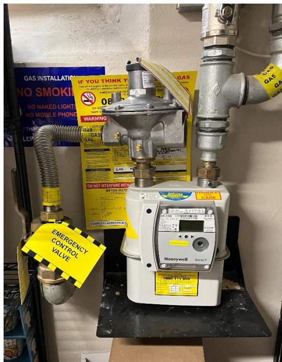
Figure 5-2 Gas meter located in store off Introduction Area
