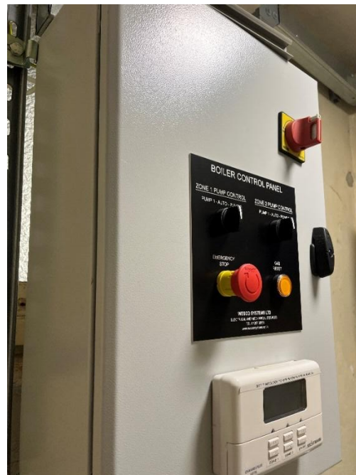
Figure 5-5 Boiler & pump control panel
